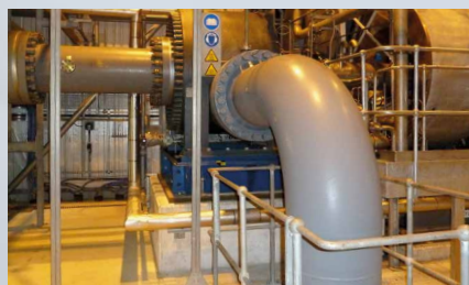
Compressor in operation at Nether Kellet Booster Station
